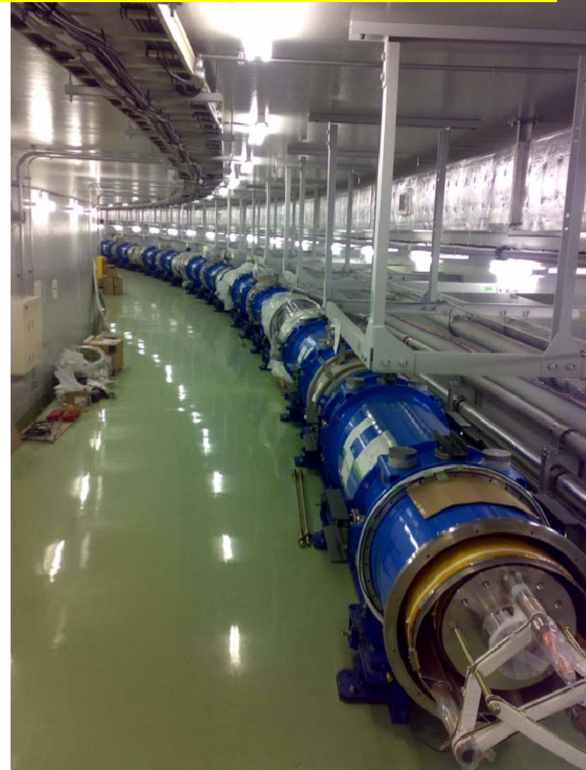
Superconducting magnets (doublet) in Tunnel
